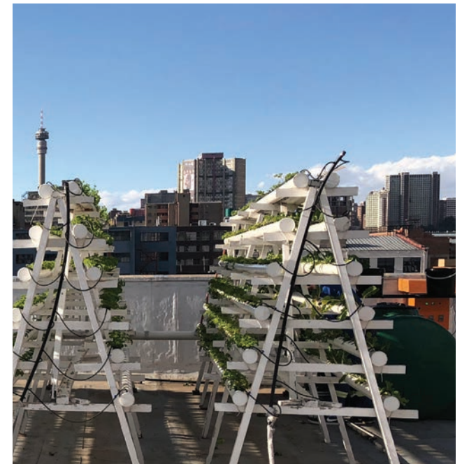
Off-grid rooftop installation powers water pump for vertical garden
