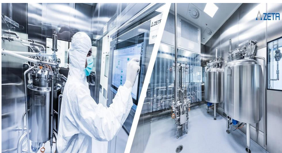
Figure 4: Advanced cleanroom design: software controlled HVAC
